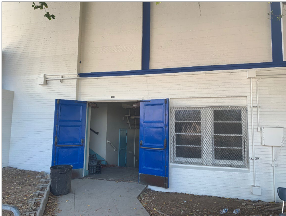
Figure 36. Entrance on the southwest façade at lower level, view toward the northeast.
