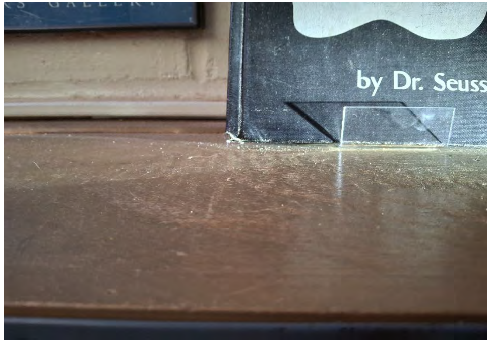
Photograph 10: View of the book shelves in the Library of Building A. Visible smoke/fire debris.
