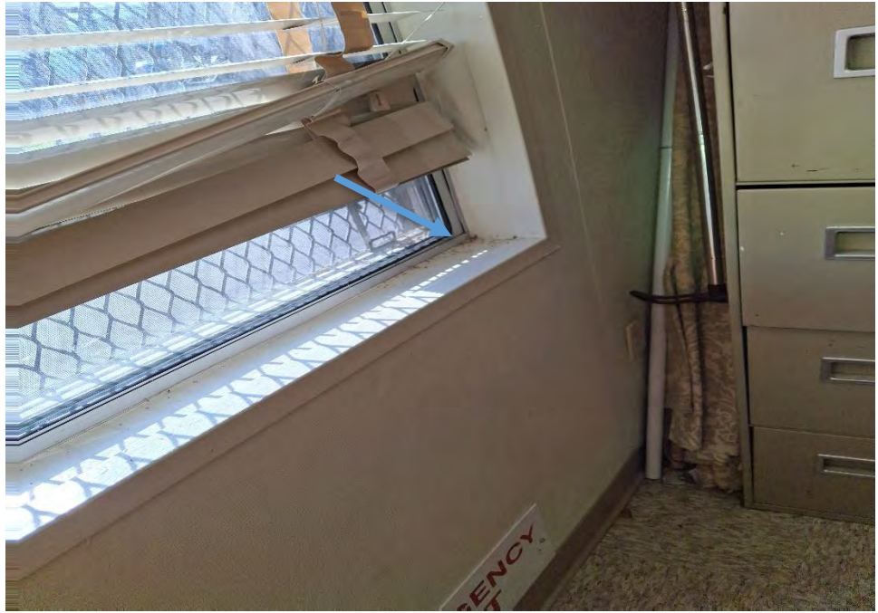
Photograph 5: View of DOH building window sills. Visible smoke/fire debris.
