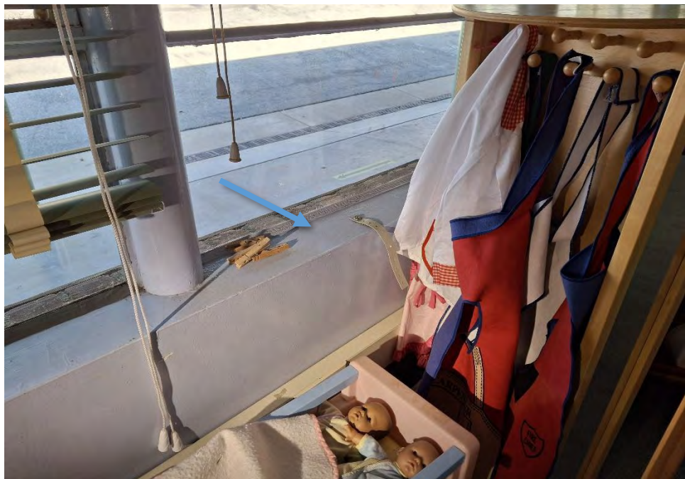
Photograph 8: View of the window sills in the Main Building classroom. Visible smoke/fire debris
