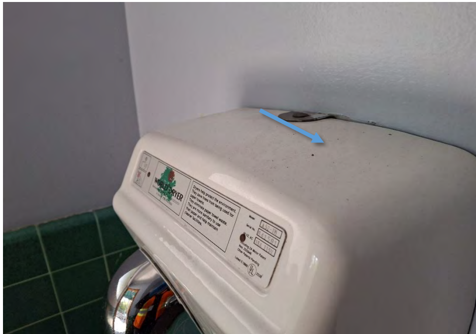
Photograph 11: View of the hand dryer in Building B. Visible smoke/fire debris.
