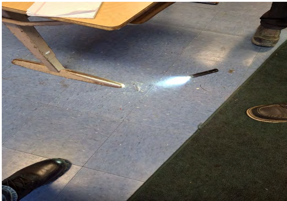
Photograph 2: View of the floor in Building AA-4088. Visible smoke/fire debris.
