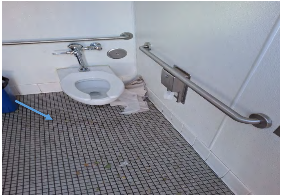
Photograph 6: View of the New Sanitary Building. Visible smoke/fire debris.
