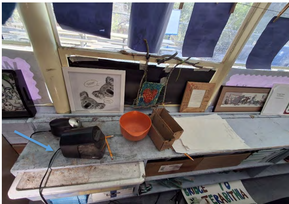
Photograph 12: View of low shelves in Building B. Visible smoke/fire debris.
