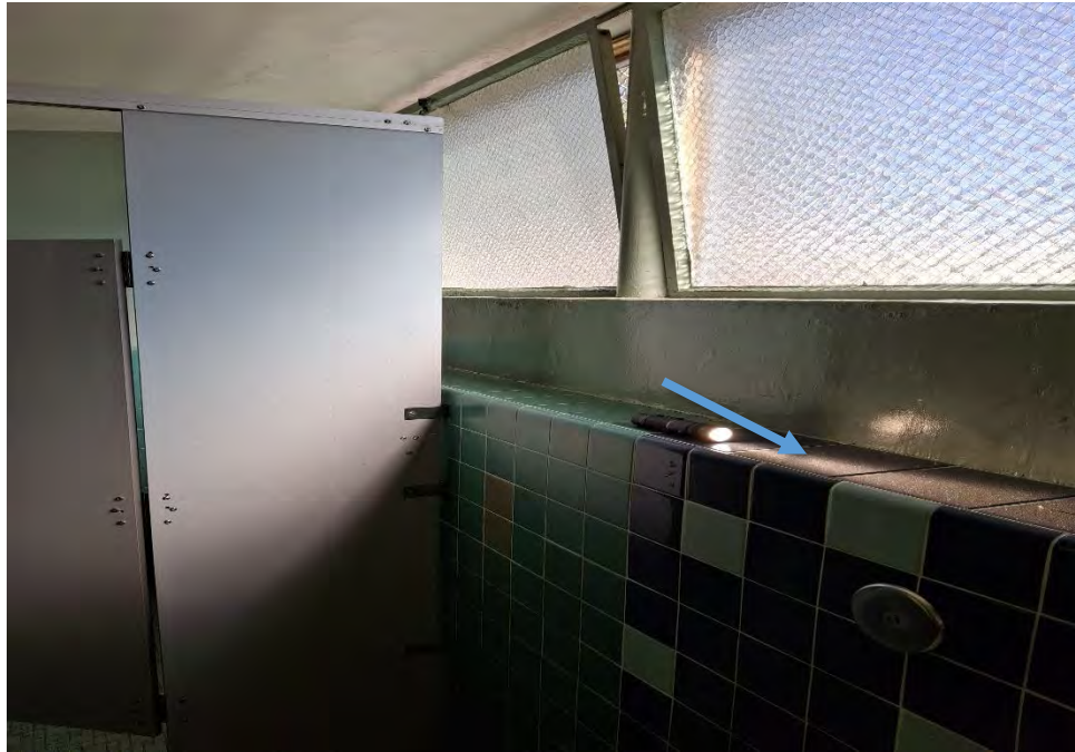
Photograph 15: View of Building D out of order restrooms. Visible open window, and smoke/fire debris
