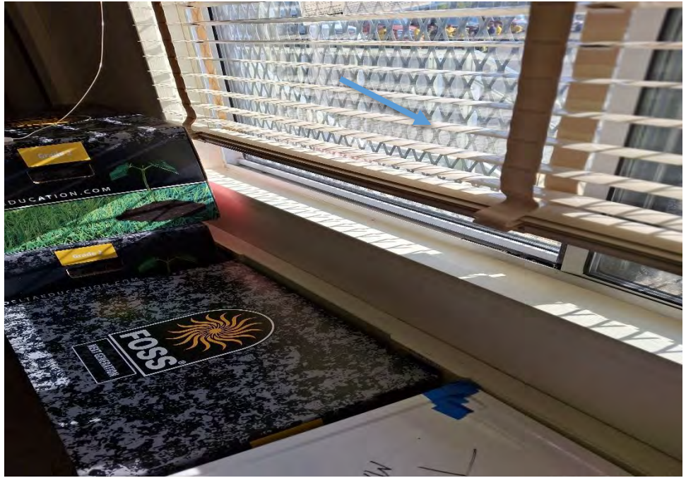
Photograph 3: View of the blinds in building AA-4087. Minor Visible smoke/ fire debris.
